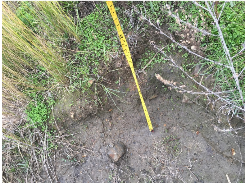
Figure 4 - Minor erosion on side slope
